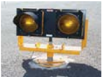
Figure 2. Embedded Runway Guard Light
